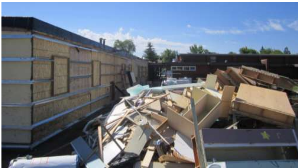
Summer of 2011 – rubble removed from inside the old building is piled in the old court yard. To the left, the exterior of the renovated section is readied for the new look.
