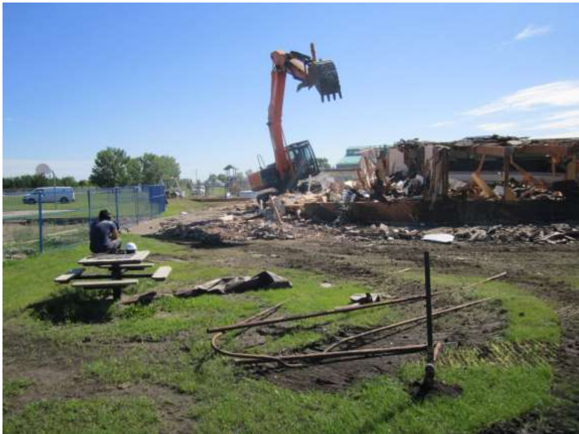
July 2011 – The crane begins the demolition of the 1950's west wing of old Duclos School.
