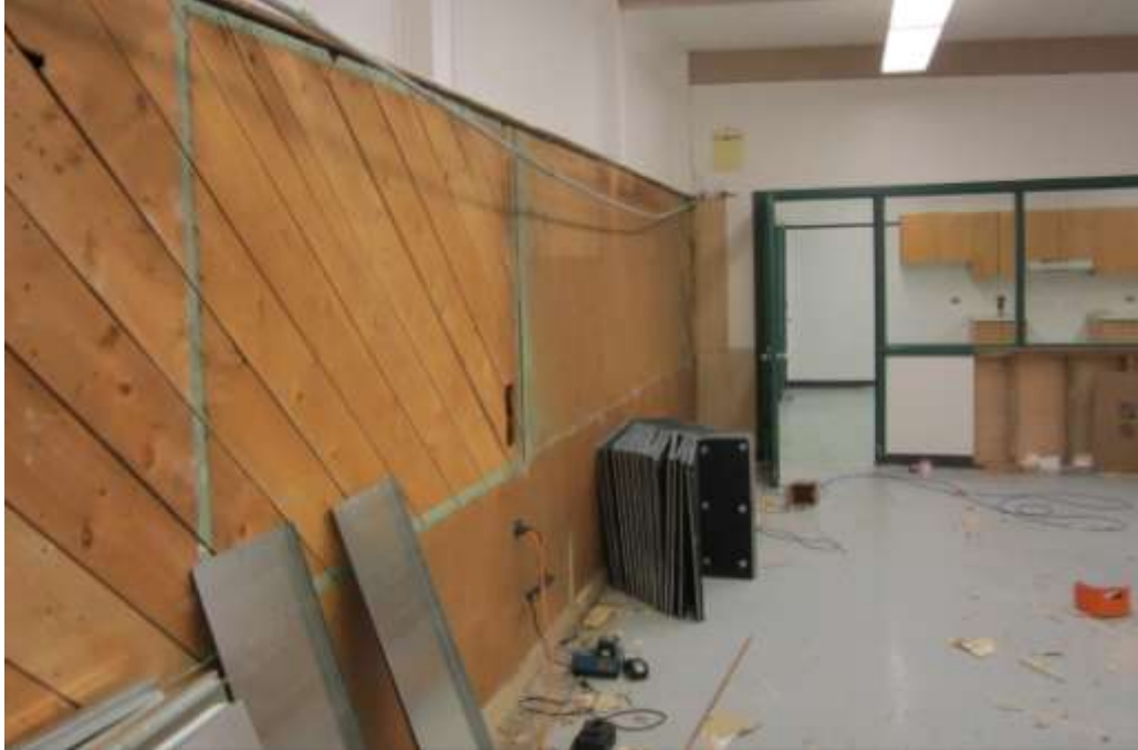
Summer of 2011 – Inside the renovation of the old building – stripping away the old walls.
