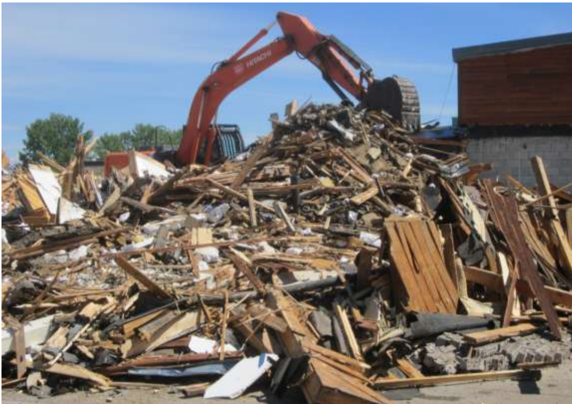
July 2011 - The crane is moving in to begin to knock down the old Duclos gym.
