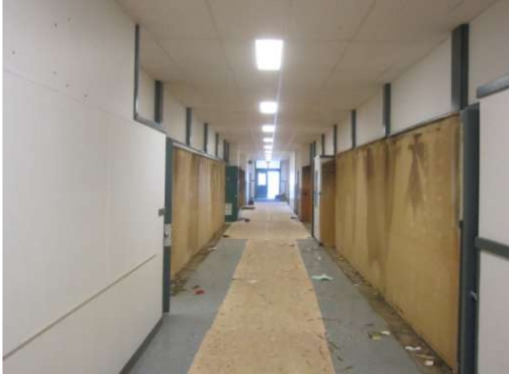
Summer 2011 – the old junior high hallway is stripped and readied for new flooring, walls, paint, and lockers.
